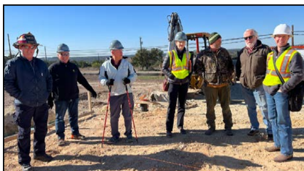
Chief Zimmerman and the Building Committee meet weekly on-site with the architect and general contractor.
